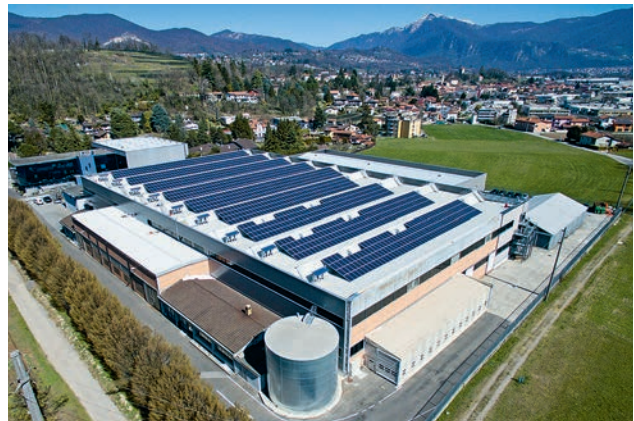
Commissioned in 2015: naturemade star-certified photovoltaic plant of the energy suppliers Azienda Elettrica Ticinese and Aziende Municipalizzate di Stabio in Stabio TI. (Photo: AET)
